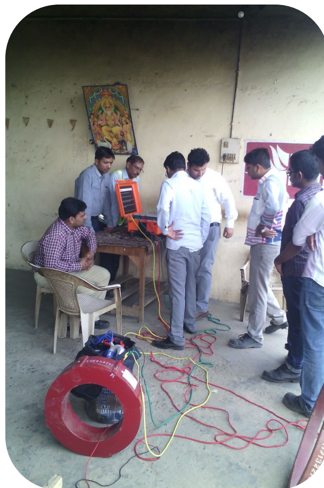
6000:1 Generator Bus Duct CT
