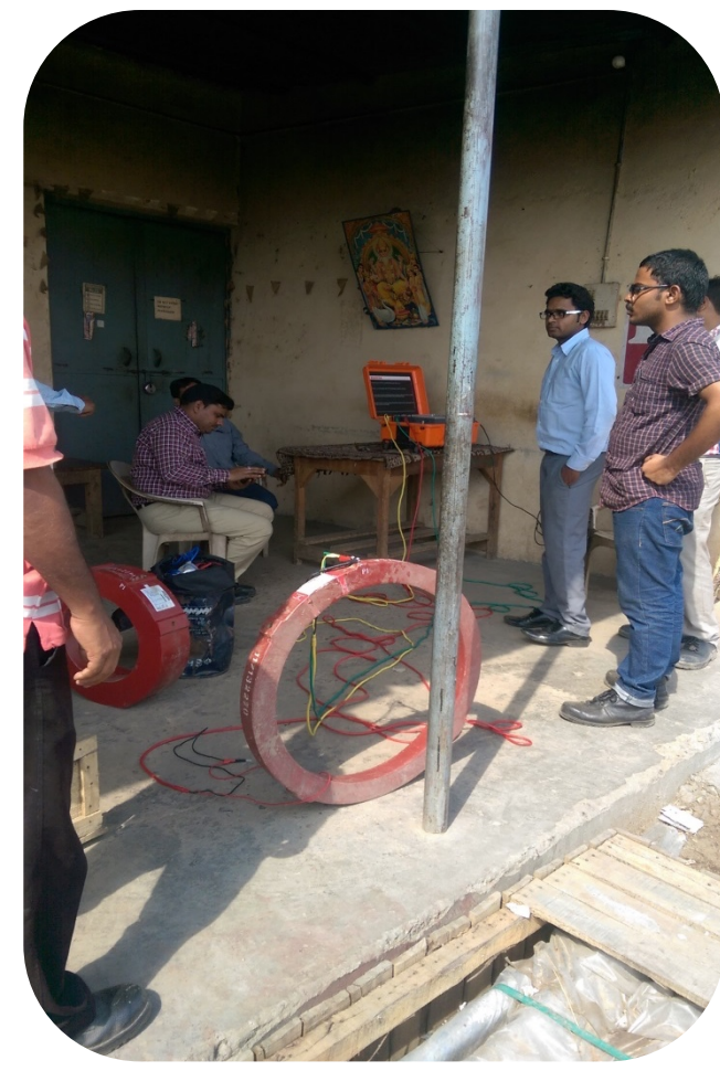
8000:1 , Generator Bus Duct CT
