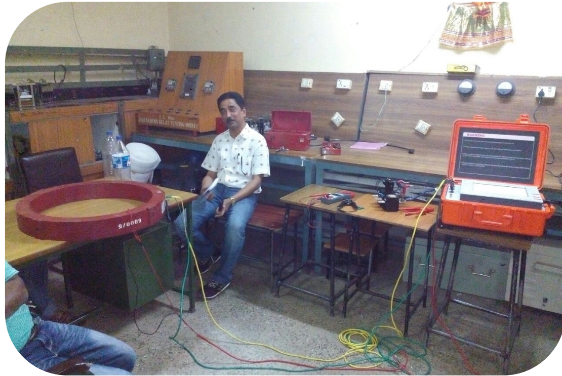
6000:1 Generator Bus Duct CT
