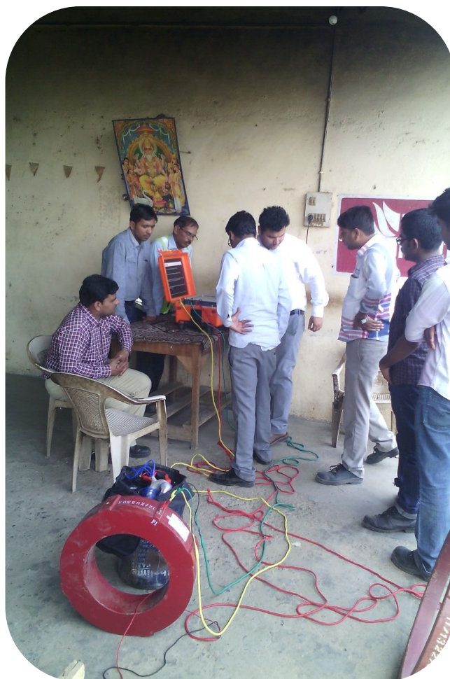
6000:1 Generator Bus Duct CT
