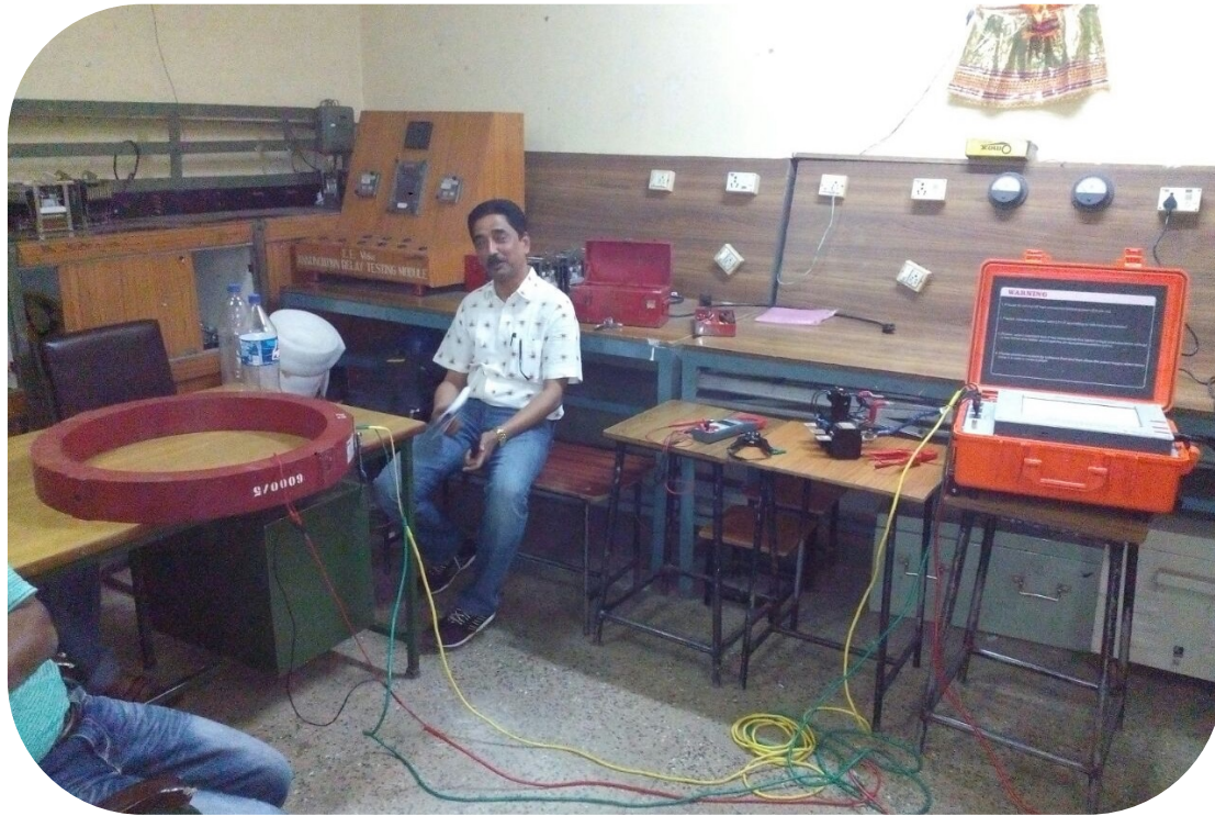
6000:1 Generator Bus Duct CT
