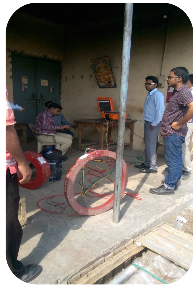
8000:1 , Generator Bus Duct CT
