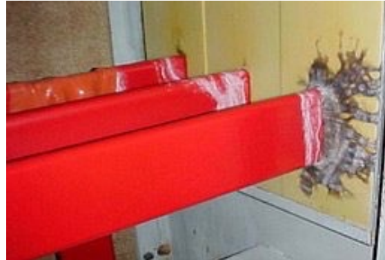
Partial discharge In Busbar Insulation
